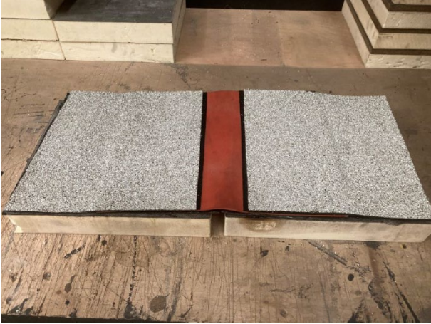
7) Ensure care is taken to avoid directly torching the joint ( temporary protection of exposed joint )
