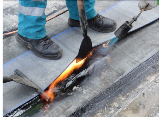
8) The waterproofing cap sheet is torch bonded to the upper side of the joint
